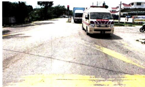
Faded road lines at the Jalan Teluk Pulai and Jalan Mengkuang intersection, where accidents often occur.
